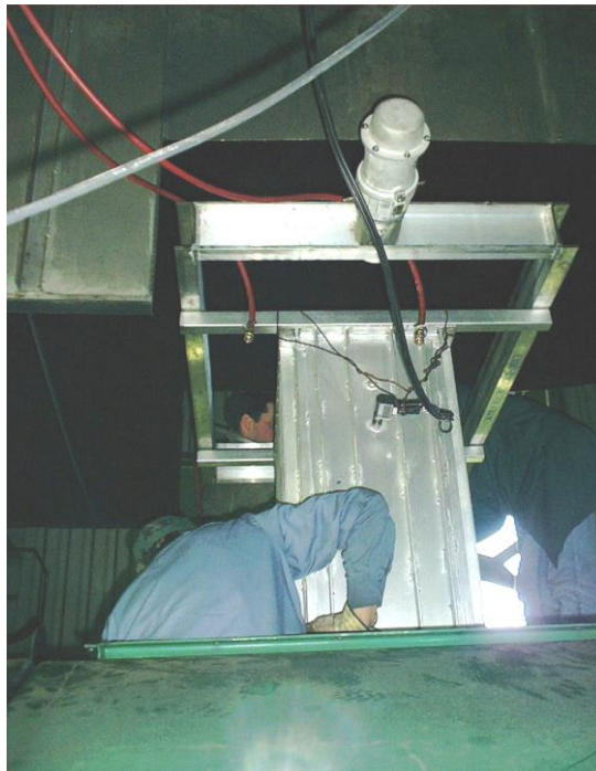
Figure 2. Exhaust Stack Extension and Sampling Systems
